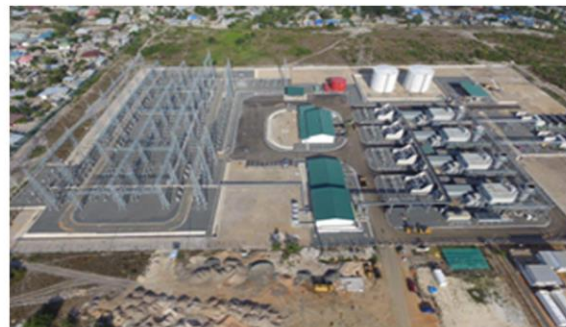
Gas Fired Power Plant
